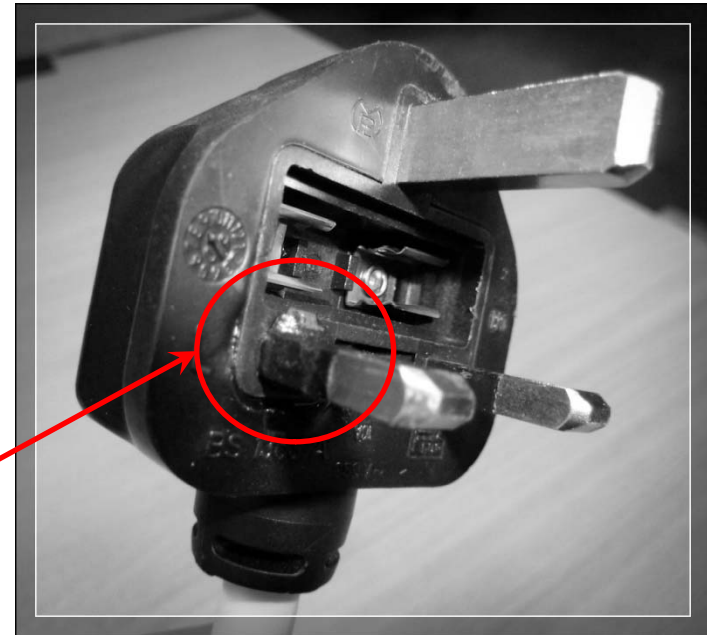
Damage to BS1363 plug due to use in EV charging Source: ESB
