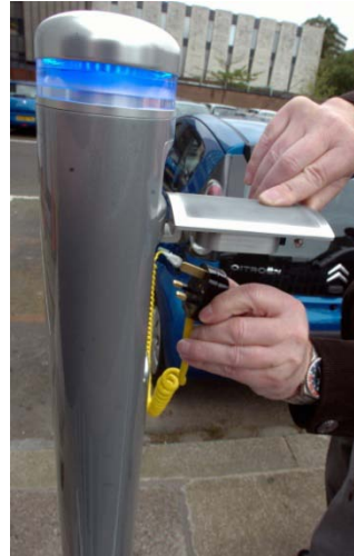
1 of the charging points in use at the Civic Centre
